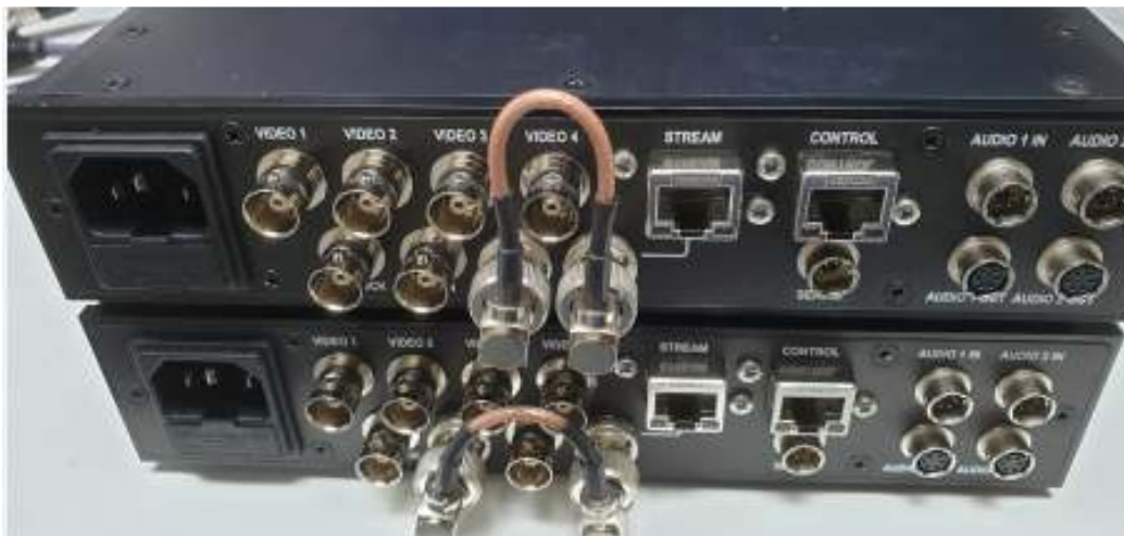
ASI Link Cable Fitted to Sapphire HEVC Encoder
